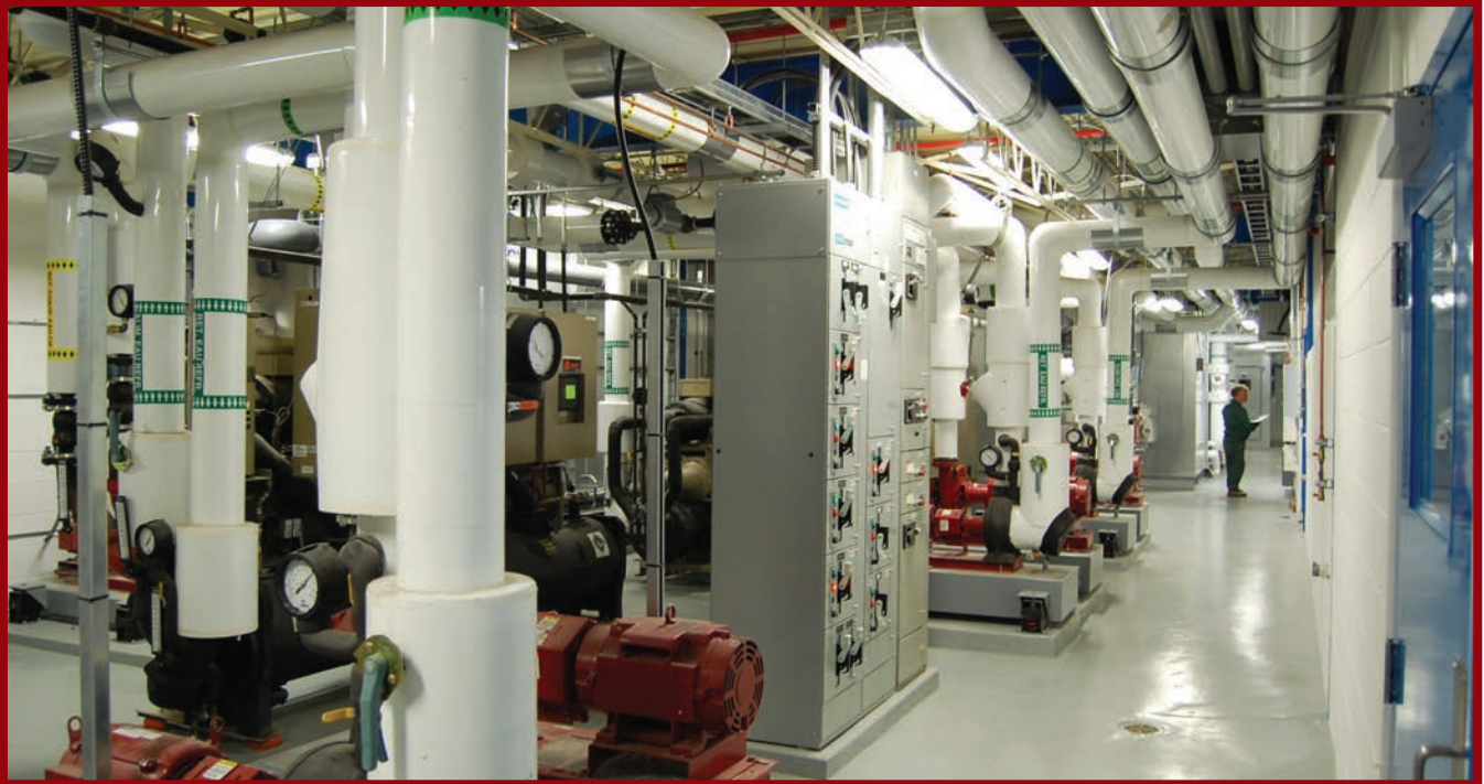
Mechanical mezzanine at Buanderie Centrale de Montreal, a laundry that underwent a major retrofit that saves $300,000 annually.
